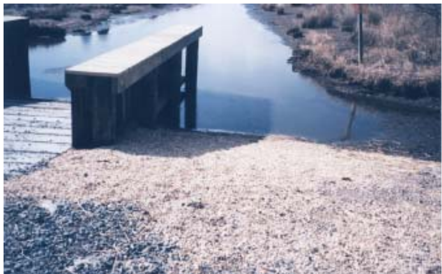
Photos 11B: Geocell material anchored with pea gravel offers low-impact access while helping to stabilize an eroding bank
